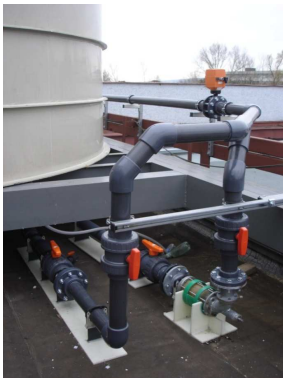
Figure 4. Pumping power plant at Faculty of Electrical Engineering and Information Technology of Slovak University of Technology
